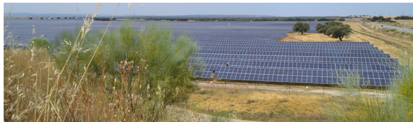
Solar plant in Spain, 300 MW.
