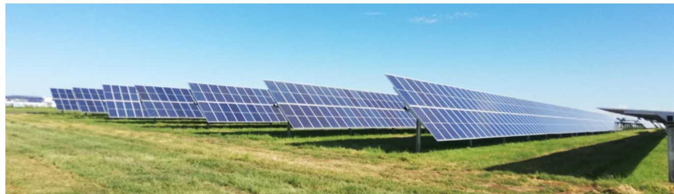
Solar plant in Australia, 70 MW.
