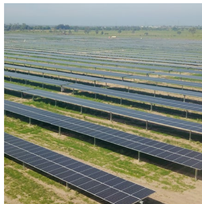
Solar plant in Spain, 50 MW.
