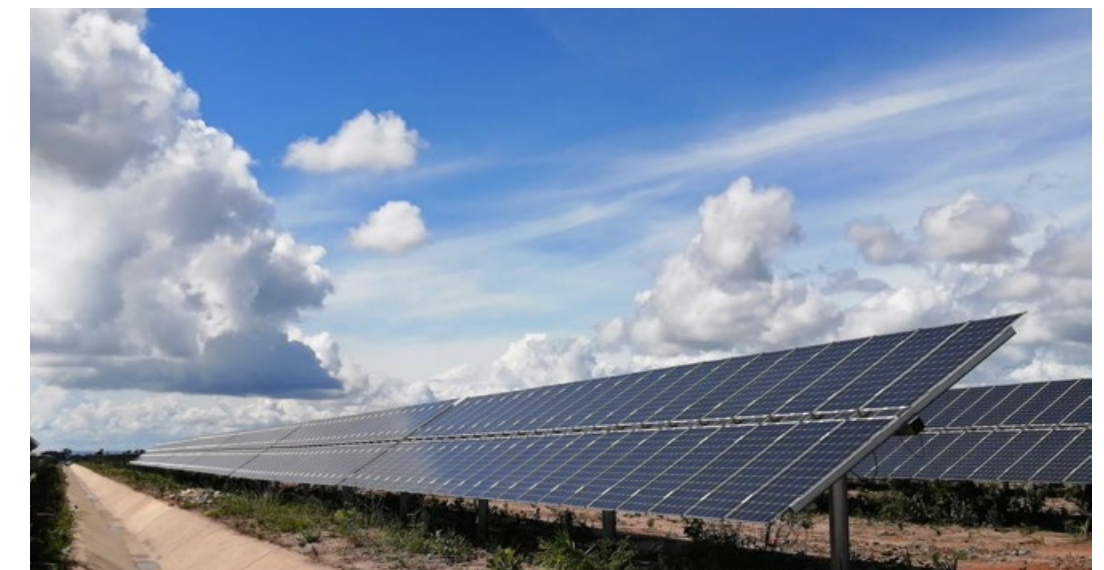
Solar plant in Spain, 5 MW.
