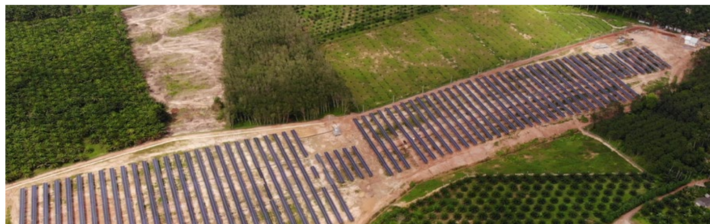
Solar plant in Thailand, 10 MW.
