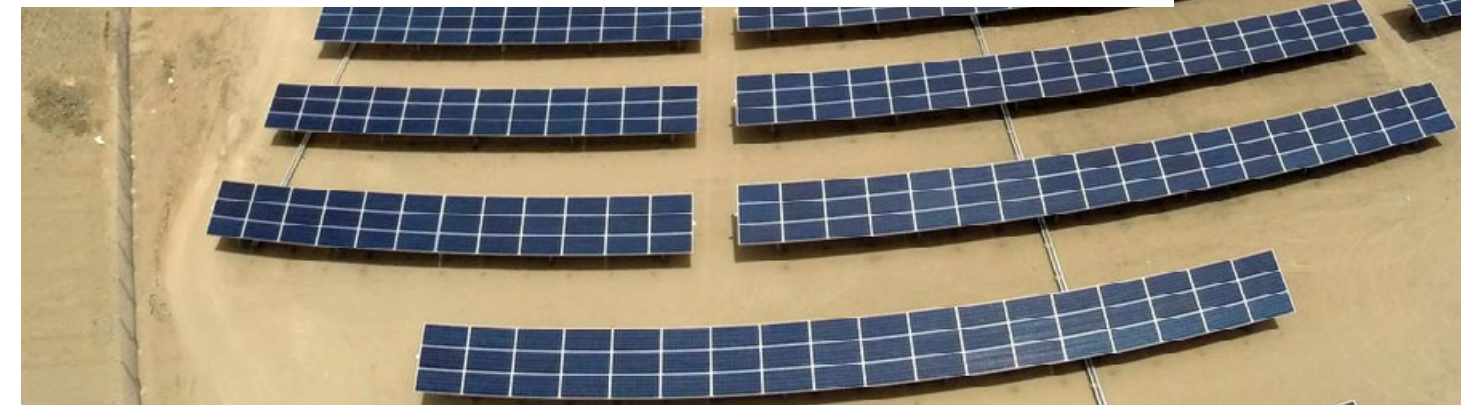
Solar plant in Chile, 12 MW.
