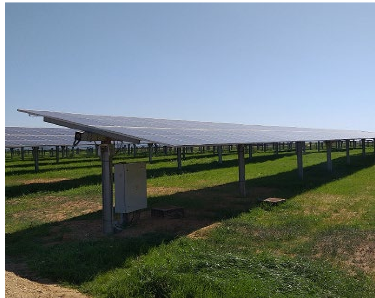
Solar plant in Spain, 50 MW.
