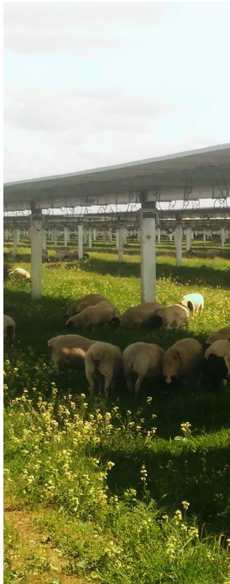
Solar plant in Australia, 70 MW.
