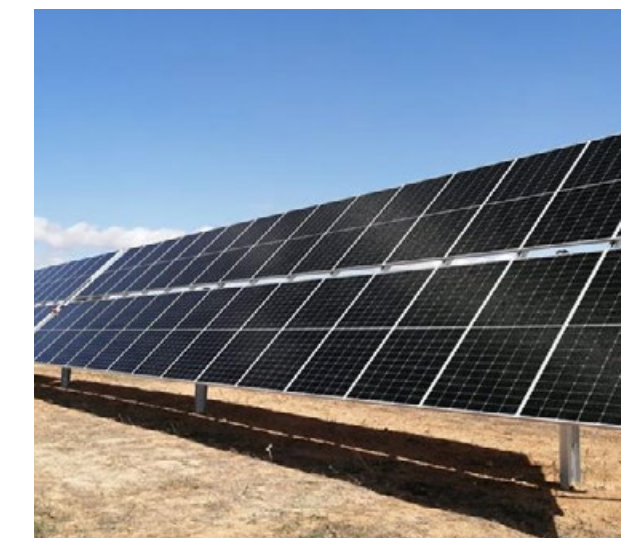
Solar plant in Spain, 5 MW.
