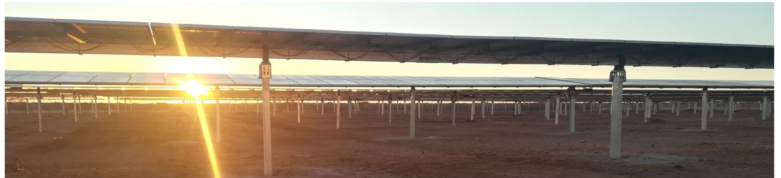
Solar plant in Namibia, 48MW
