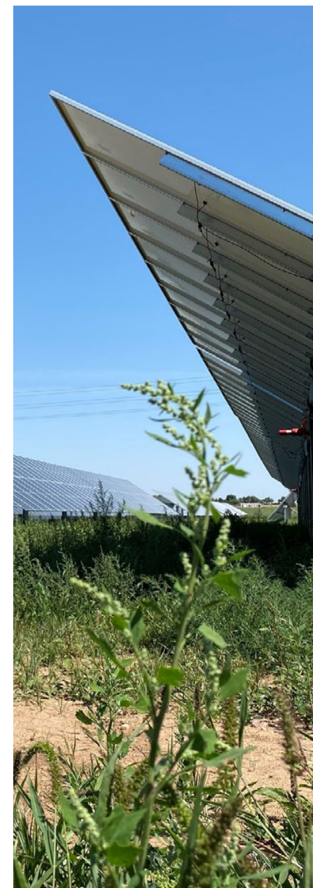
Solar plant in Spain, 5 MW.
