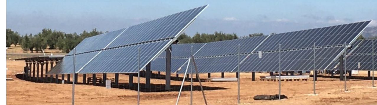
Solar plant in Spain, 5 MW.
