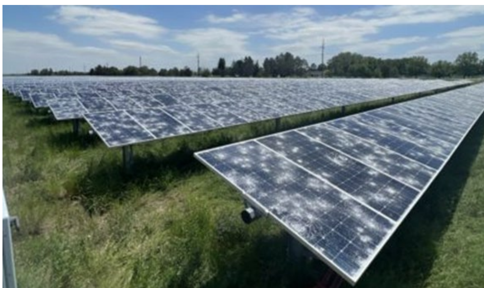
Figure 3. Hail damage on photovoltaic solar tracking facilities.
