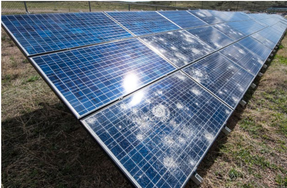
Figure 2. Hail damage on fixed photovoltaic facilities.
